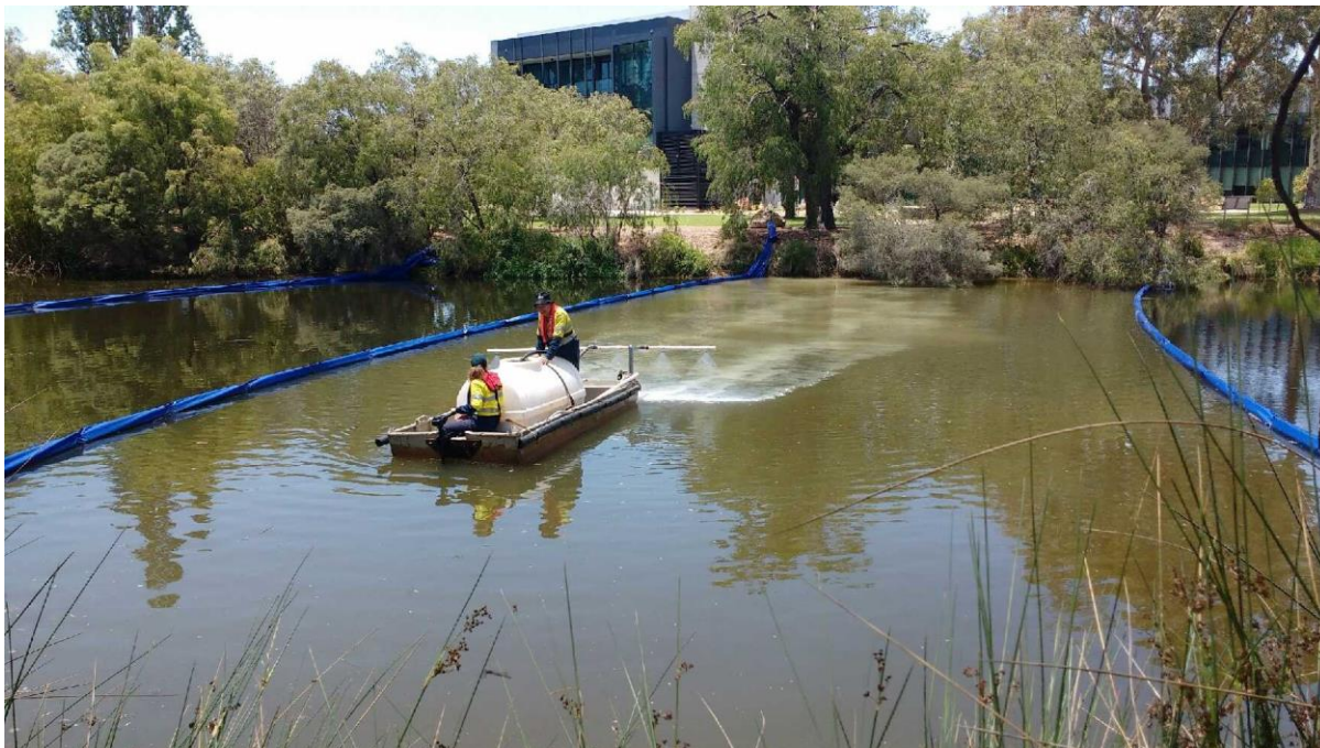
Figure 18. HT clay being applied in the Lower Vasse River during the 2017-18 trial.
